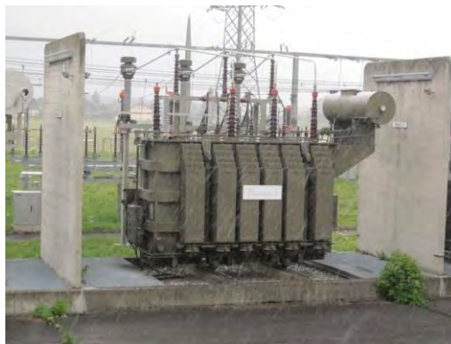
110/30-kV-Umspanner UW Lungau, 32 MVA
