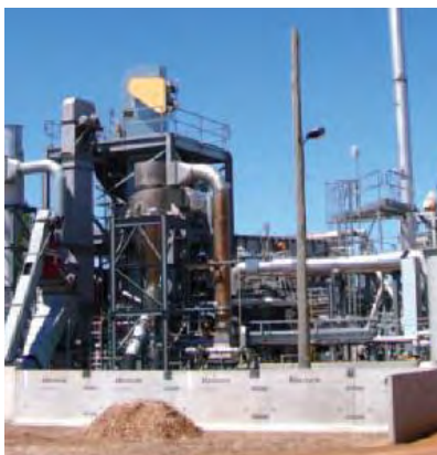
A biomass-fired power plant
