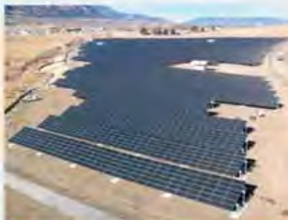
1 MW PV system of U.S. Army Fort Carson, IRE3. Photographer: Information eXchange
