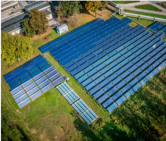
Collector test of various collector types with 3,123 m 2 for solar district heating feed-in at the district heating plant Puchstrasse in Graz, Austria; Photo: S.O.L.I.D. GmbH
