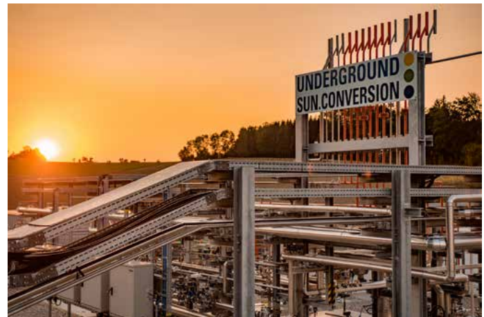
RAG facility in Pilsbach/Upper Austria, Photos: RAG Austria AG/Karin Lohberger Photography
