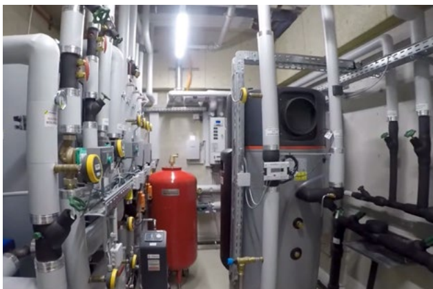
Plant room with heat pump, photo: Stadtwerke Wörgl GmbH
