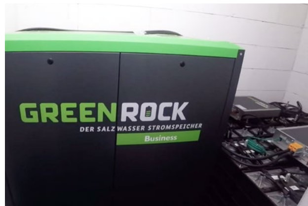
Saltwater battery storage system with 40 kWh capacity, photo: Stadtwerke Wörgl GmbH
