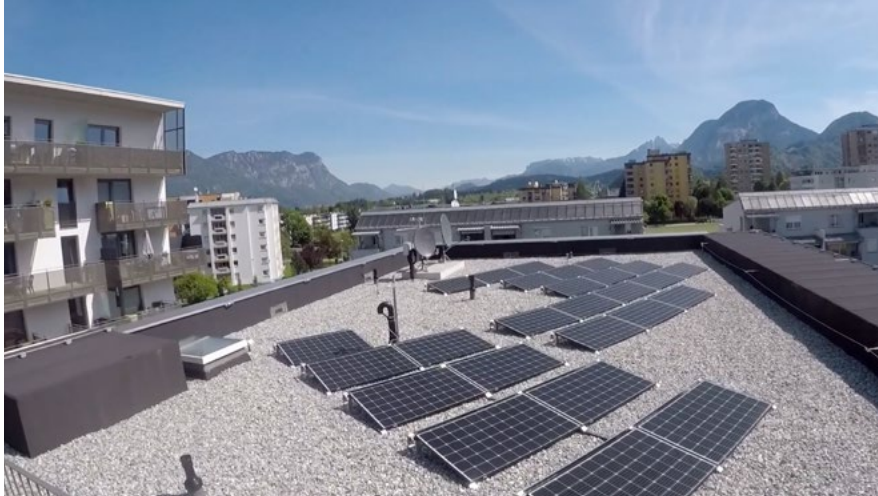
PV system with 29 kWpeak output installed on the three roofs of the first-phase buildings. Additional capacity of 40 kWpeak is planned for the second phase of construction, photo: Stadtwerke Wörgl GmbH
