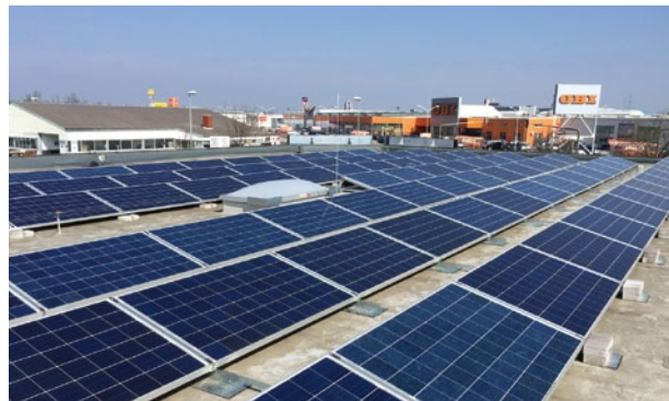
PV equipment on a supermarket building in Neusiedl am See, Photo: IEV AG
