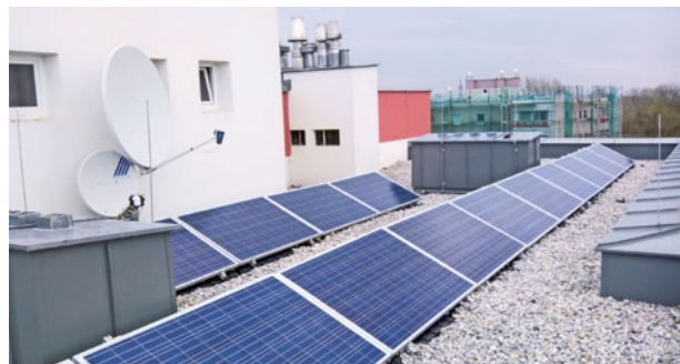
PV modules on the Porsche housing complex in Wiener Neustadt, Photo: Wien Süd
