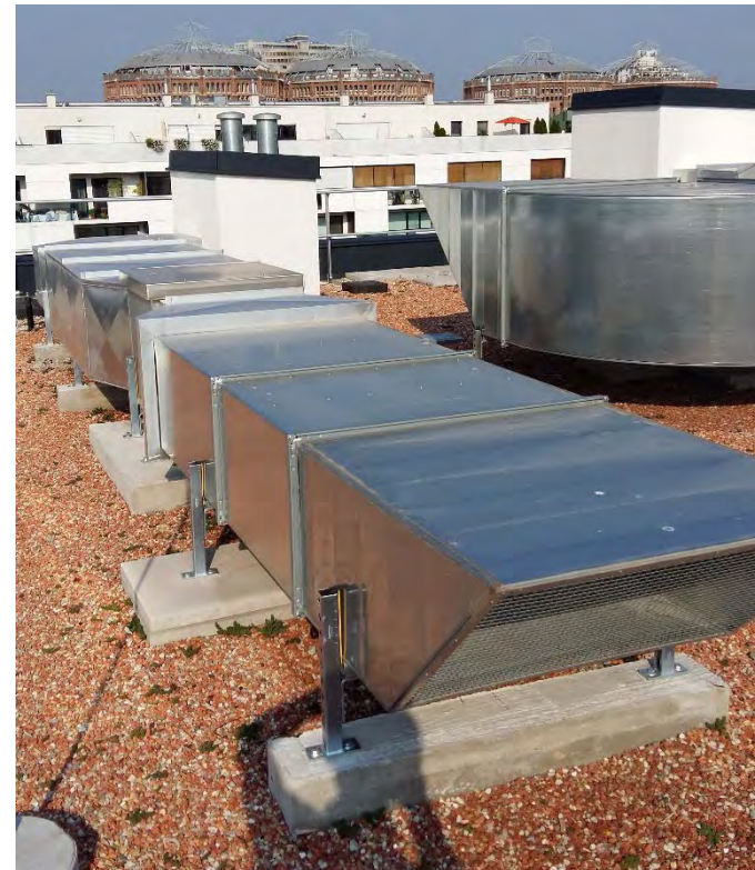
Exhaust ventilator on roof source: Peter Holzer
