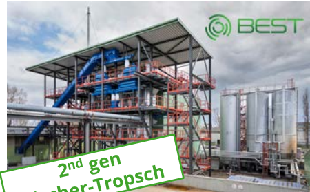
1 MW Syngas Platform Vienna
