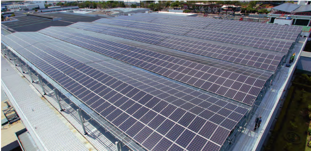
BIPV System at Bosch plant, Penang, Malaysia
