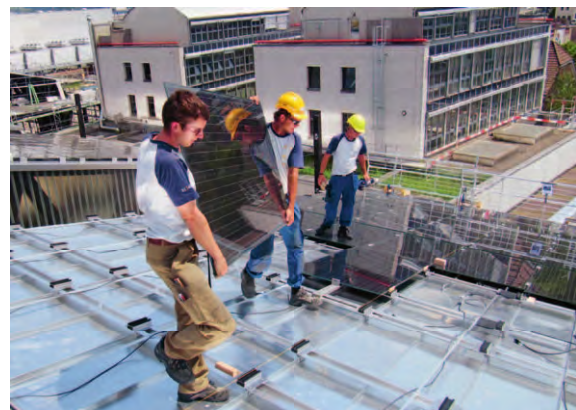
Rooftop installation in bern, Switzerland, Photo: BE Netz AG
