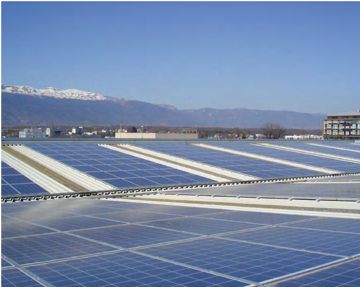
PV on a Brewery in Switzerland, Photo: ADEV Liestal
