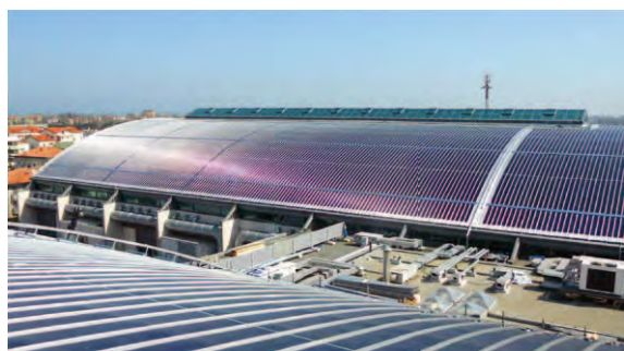
Green Utility SpA-owned Si-a 4,3 MWp PV plant, Rimini Fair, by the contractor Acea Arse SpA
