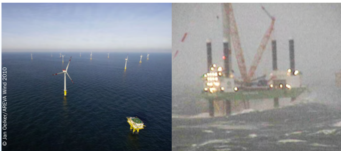
FIGURE 5 ALPHA VENTUS WIND FARM COMPLETED (LEFT) AND IN HARSH WEATHER CONDITIONS DURING CONSTRUCTION (RIGHT)
