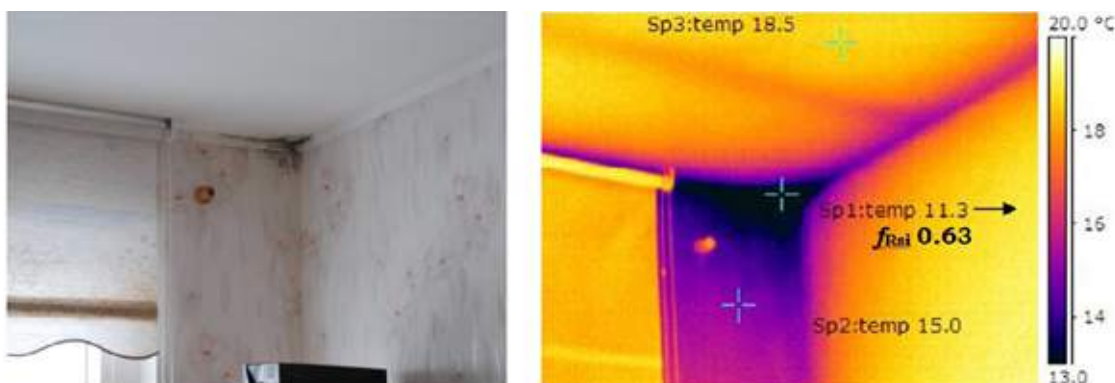
Visible mould growth at the corners of a building envelope, possibly caused by a thermal bridge.
