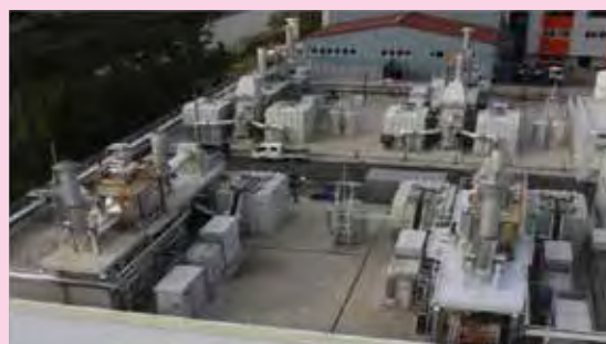
Figure 8: Daegu, 11.2MW MCFC installation in Korea
