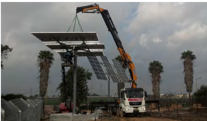
The tracking systems are installed on top of 8 m high poles in order to prevent shading. They are installed in a plant yard at Kibbutz Ein Zurim. Photo by: Ormash
