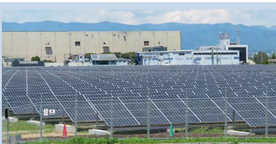
The 2.1 MW "SoftBank Kyoto Solar Park", commissioned in July 2012, is one of the first MW-scale PV plants qualifying for the new FiT programme. Photo by RTS Corporation.
