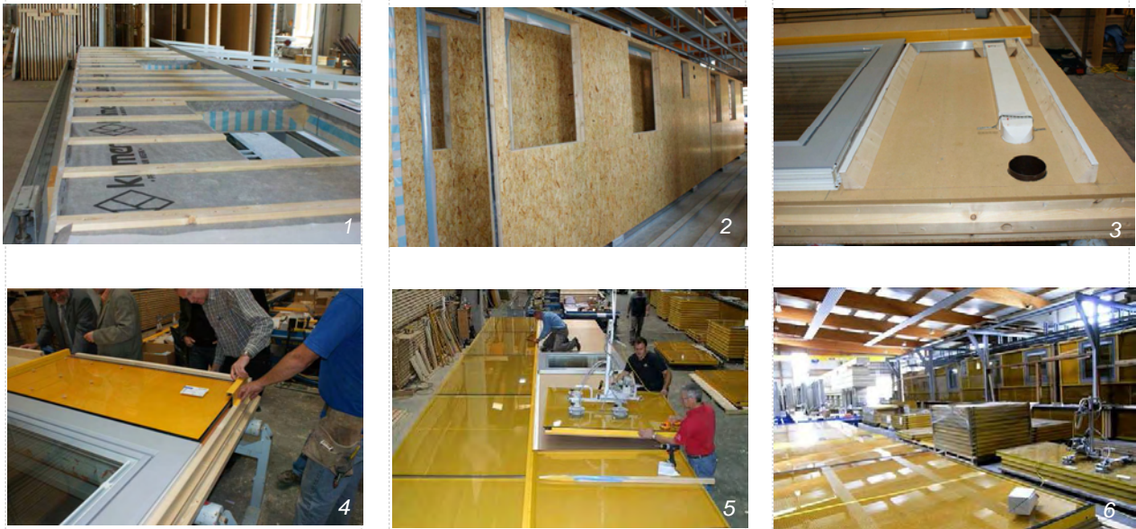
Figure 14: Sequence of pre-fabrication procedure in the fabrication hall [Source pictures 5-6: Gap-Solution GmbH]
