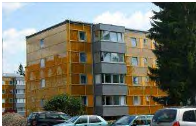
Picture 3-4: Integrated balconies after renovation within residential area Dieselweg, Graz (Source: AEE INTEC)
