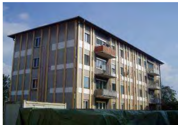
Picture 8-2: Levelling laths made of a timber substructure. Example: Dieselweg, Graz (Source: AEE INTEC)
