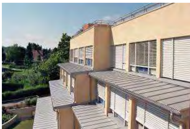
Picture 3-1: South-west oriented windows – shadowed with exterior blinds (Source: Ziv.Ing. Büro Boder)
