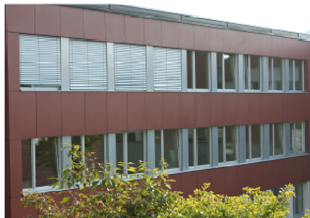
Picture 3-2: South-east oriented class-room windows – shadowed with exterior blinds (Source: AEE INTEC)
