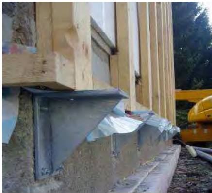
Picture 8-1: Steel angles as support brackets at the bottom. Example: Dieselweg Graz (Source: AEE INTEC)
