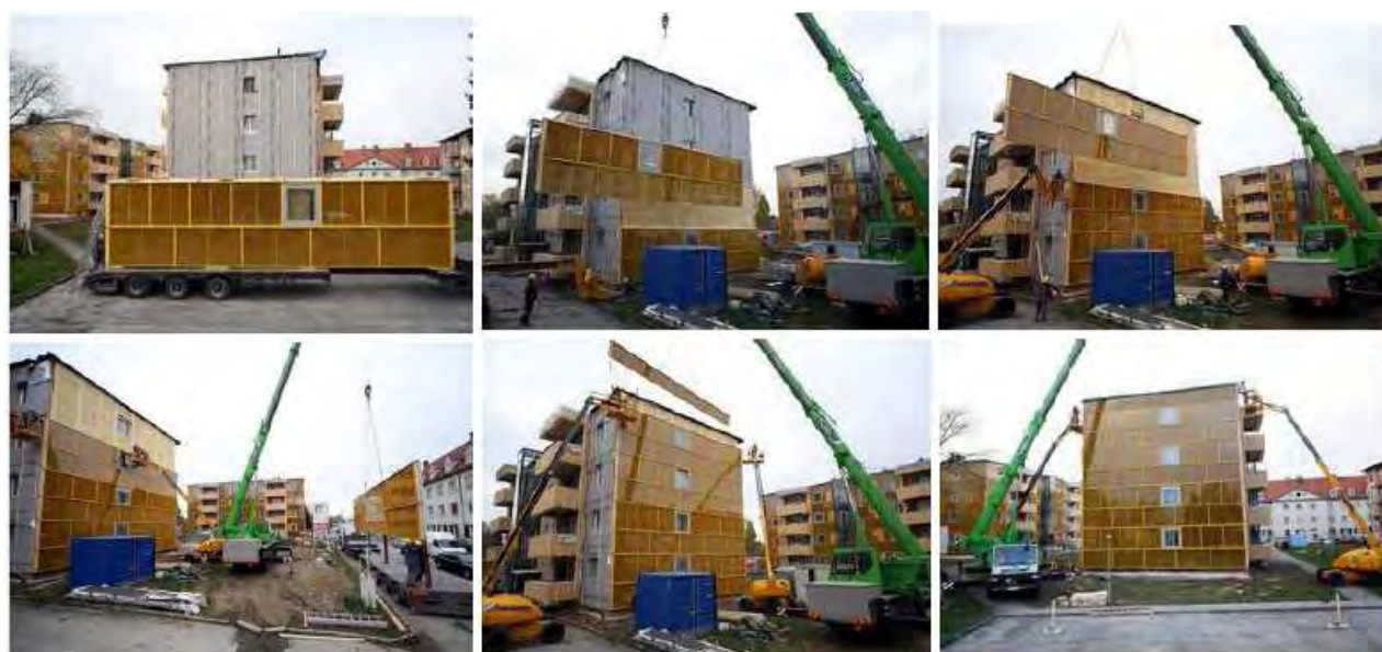
Picture 1-2: Assembling procedure of pre-fabricated façade modules within the renovation “Dieselweg”, Graz-Liebenau (Source: gap-solution)
