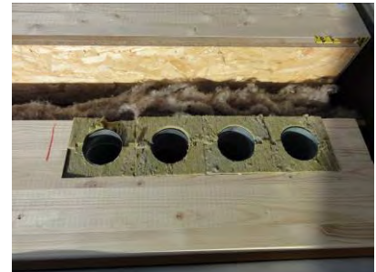
Figure 11: The ventilation ducts are fire protected with specially designed mineral wool sections.
