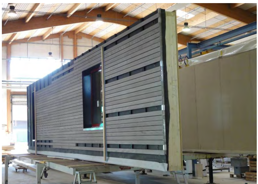
Figure 15: The windows and the wood cladding are installed, except for areas where the module has to be fixed on site
