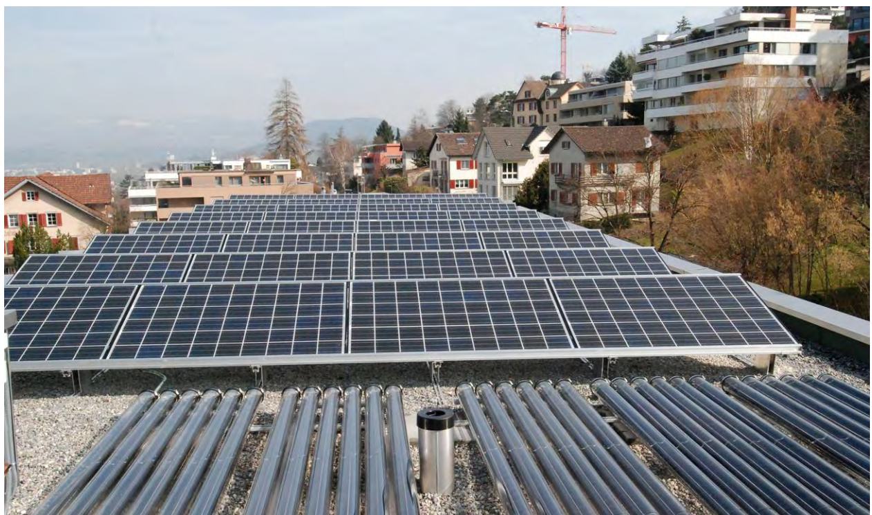
Figure 11: Thermal and PV-collectors on the roof reduce the yearly energy consumption close to zero
