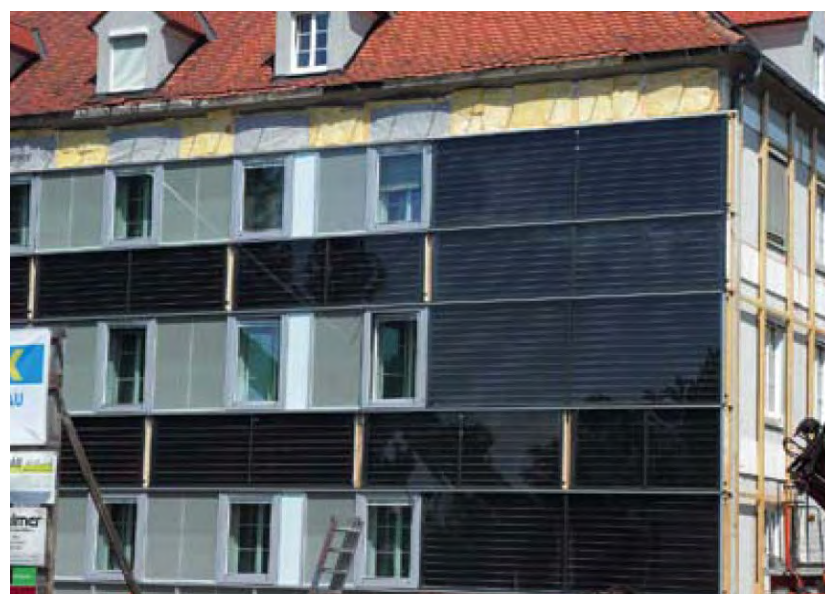
Figures 20-22: Sequence of assembly of the modules on the south-oriented façade (Source: Gap-Solution GmbH)
