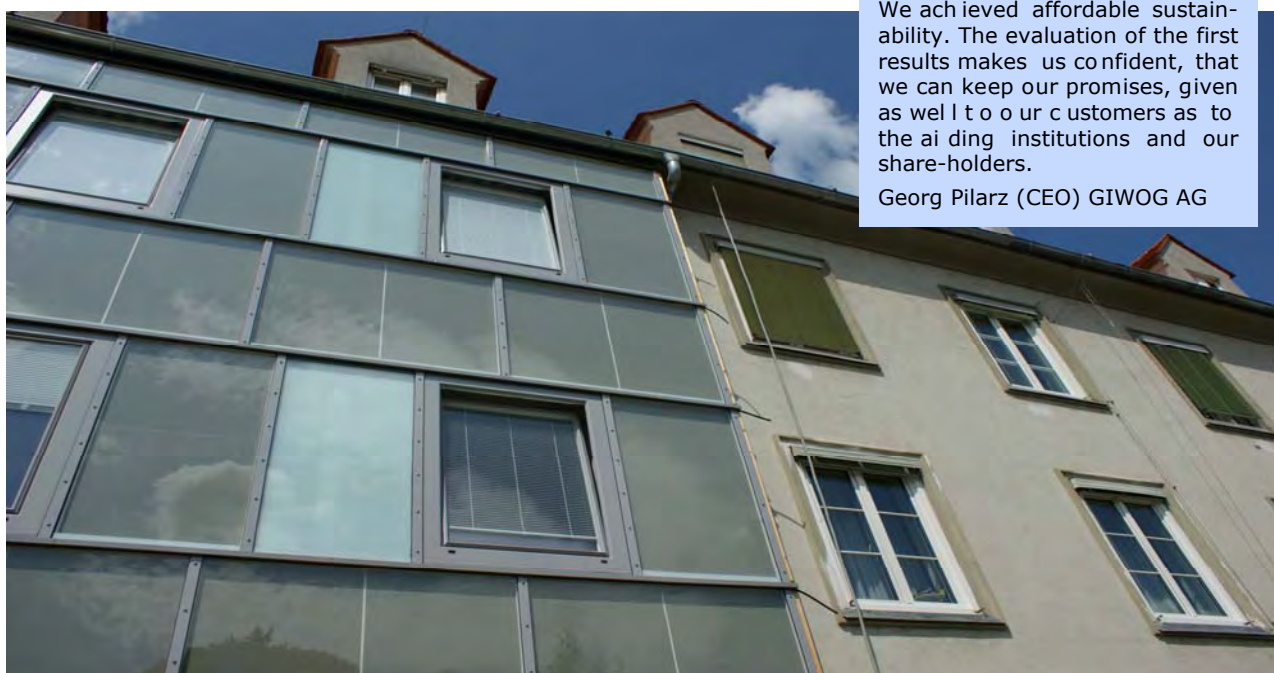
Figure 25: View on a renovated part (left) and a non renovated part of the façade (right)
