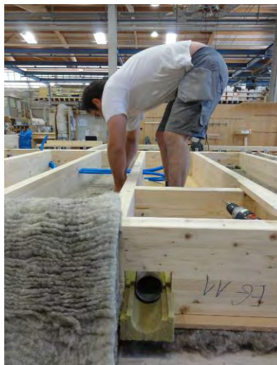
Figure 12: The timber frame construction is filled with sheep wool after the ventilation pipes and electric conduits have been mounted.
