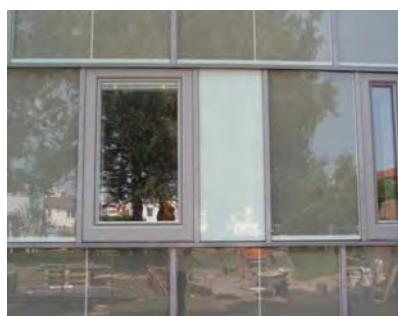
Figure 13: Window with integrated shading device and opaque field beside the window, covering supply and exhaust air ducts for ventilation
