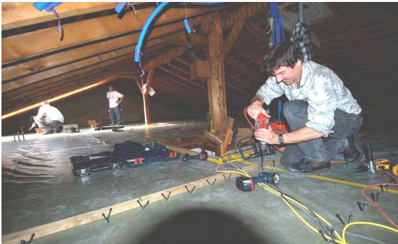
Figure 19: Mounting of reinforcement screws of the combined wood-concrete slab for the new attic floor
