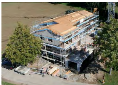
Figure 24: Areal view of the construction site, just before the façade elements were mounted (source: FHNW, René Kobler)
