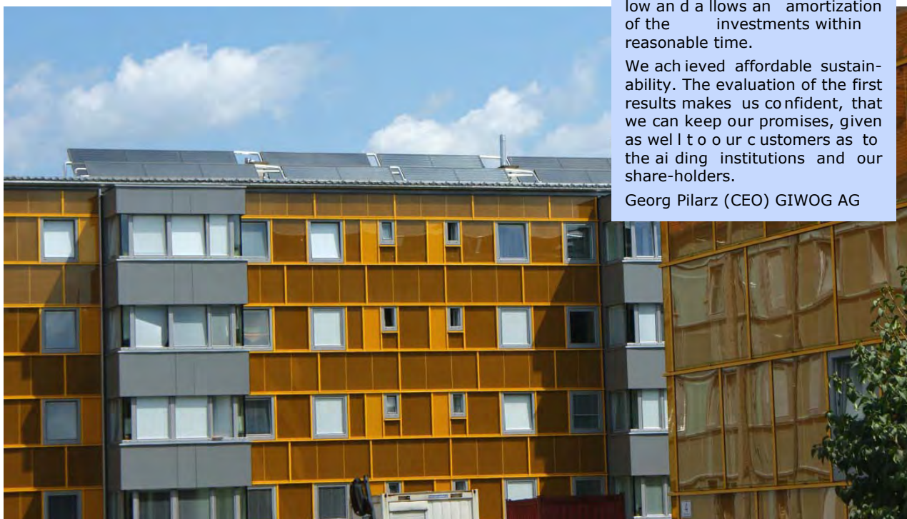
Figure 24: View on the finished façade – showing the new façade structure with integrated windows and balconies, and the solar thermal collectors on the flat roof
