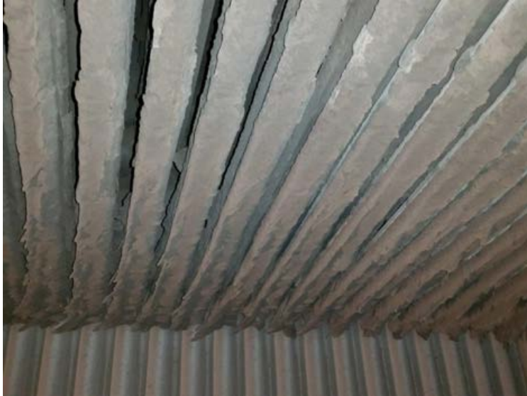
Protective evaporator from below (in the flow direction, luv) after a system operation of 9 weeks
