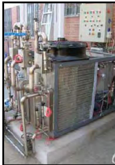
Figure 8: Air-cooled, single-double effect lithium bromide absorption chiller prototype
