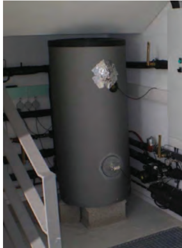
Hot storage tank of 300 liters
