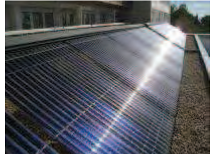
Solar collector field
