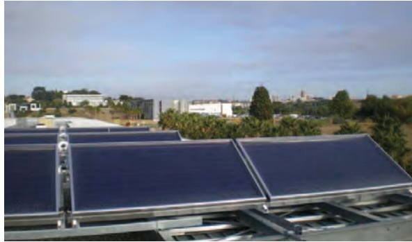
25 m 2 of double glazed solar collector
