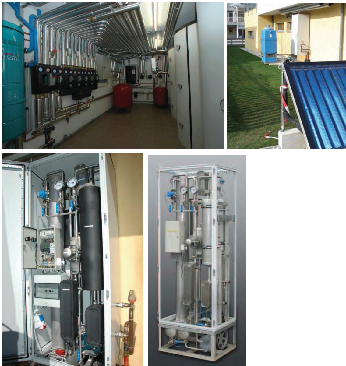
Figure 3: View of the utility room [upper left, Bachler], the outside situation with the wet cooling tower and the absorption machine [upper right, Bachler] and the inside of the cooling machine [lower left / right, Pink]
