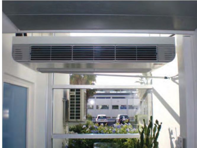
Fan coils for the distribution system
