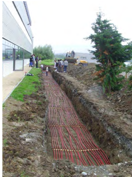
Fig. 12: Example of horizontal ground probe heat rejection system in INES office, Chambéry (source: INES RDI)
