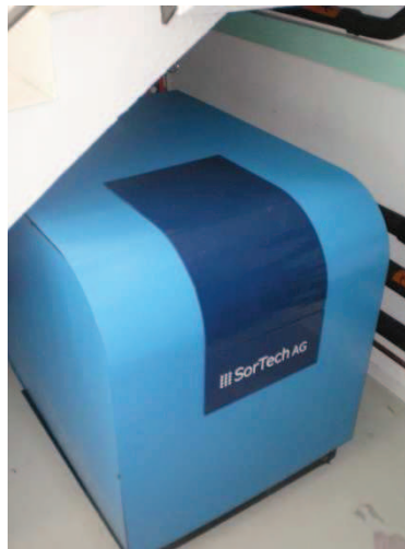
7,5 kW adsorption chiller used in Perpignan
