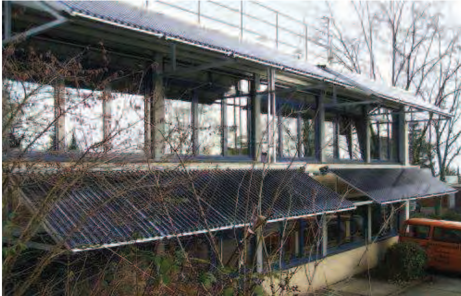
Figure 3: Evacuated tube collector field at the main building of the Technical College Butzbach. Also an effective shading of the rooms can be achieved by the assembly of the collectors. Source: Fraunhofer ISE
