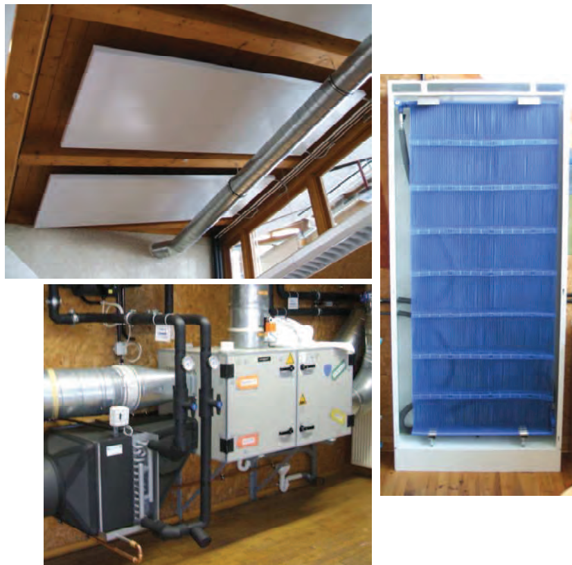
Figure 2: Cold distribution systems in the seminar rooms. Top: chilled ceiling elements; right: cooling shaft (without cover) for silent cooling and air dehumidification. Bottom: one of two air handling units with heat recovery and supply air cooling and dehumidification. The air handling unit in the seminar room was insulated additionally against acoustic noise. Source: Fraunhofer ISE
