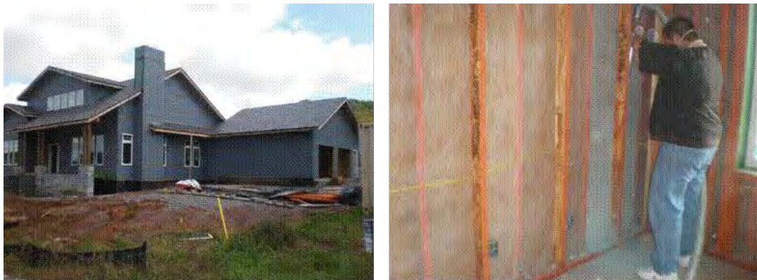
ORNL test house during construction and installation of the PCM-enhanced cellulose insulation in the double frame wall.
