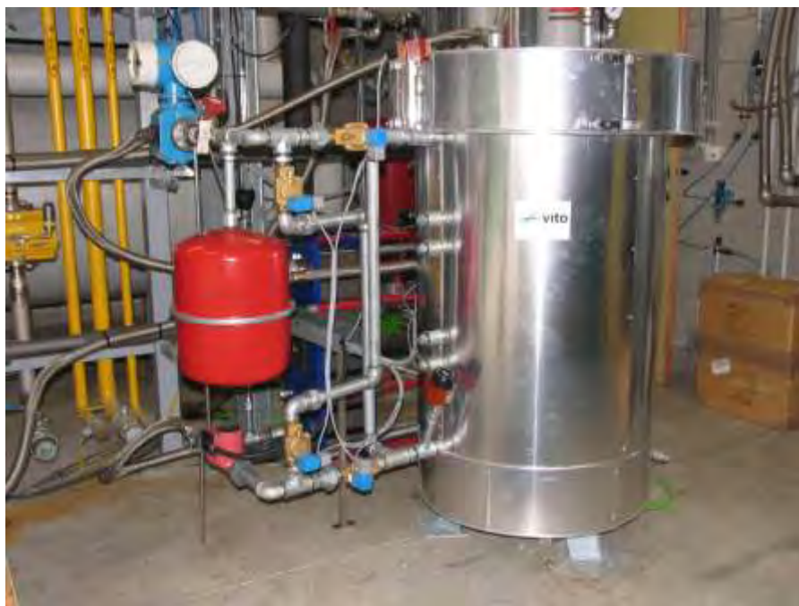
Picture of the test installation
