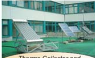
Thermo Collector and Photovoltaic-RES Laboratory
