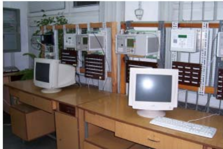
Protection relays test lab
