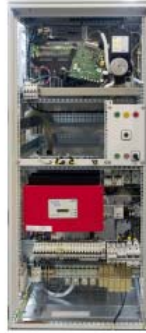
2.4 kW Fuel Cells system
