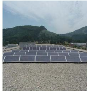
PV panels at LABEIN's roof
