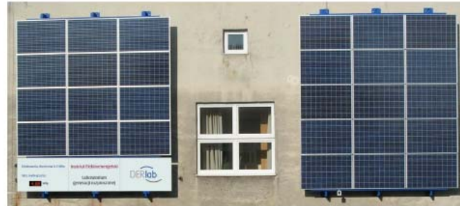
6.5 kWp PV panels on Institute of Electrical Power Engineering elevation
