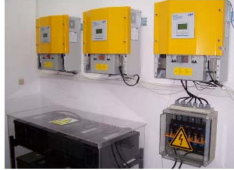
12 kW Battery storage with Sunny Islands inverters
