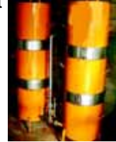
2-column system for H 2 S scrubbing with iron oxide
