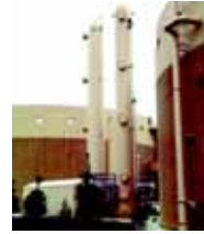
Renton plant Seattle, USA 4000 m 3 /day
