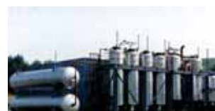
PSA unit for biogas, for \text{H}_2\text{S} , halogenated carbons, and \text{CO}_2 removal
