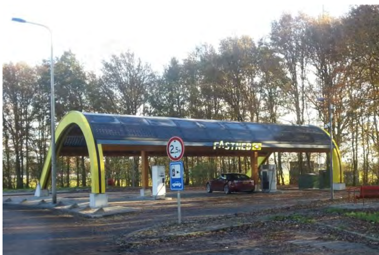
Fig. 24.2 FastNed quick charging station along Dutch highway. (Source: FastNed)
