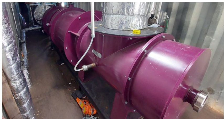
Pyrolysis gas cooler and gas burner at the test facility, photo: BIOS BIOENERGIESYSTEME GmbH
