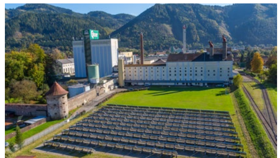
③ Solar process heat at Göss brewery (2014) – The mashing process was converted and a 1,470 m 2 solar thermal collector now supplies hot water in a low-temperature process thanks to a new heat exchanger – an Austrian contribution to IEA SHC Task 49 Solar Heat Integration in Industrial Processes. (Photo: AEE INTEC)
