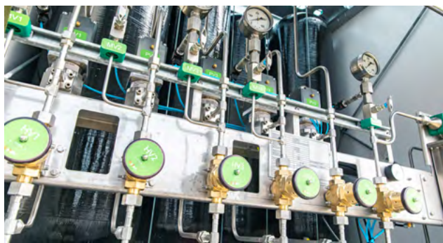
Renewable Gasfield, Photo: Energie Steiermark
