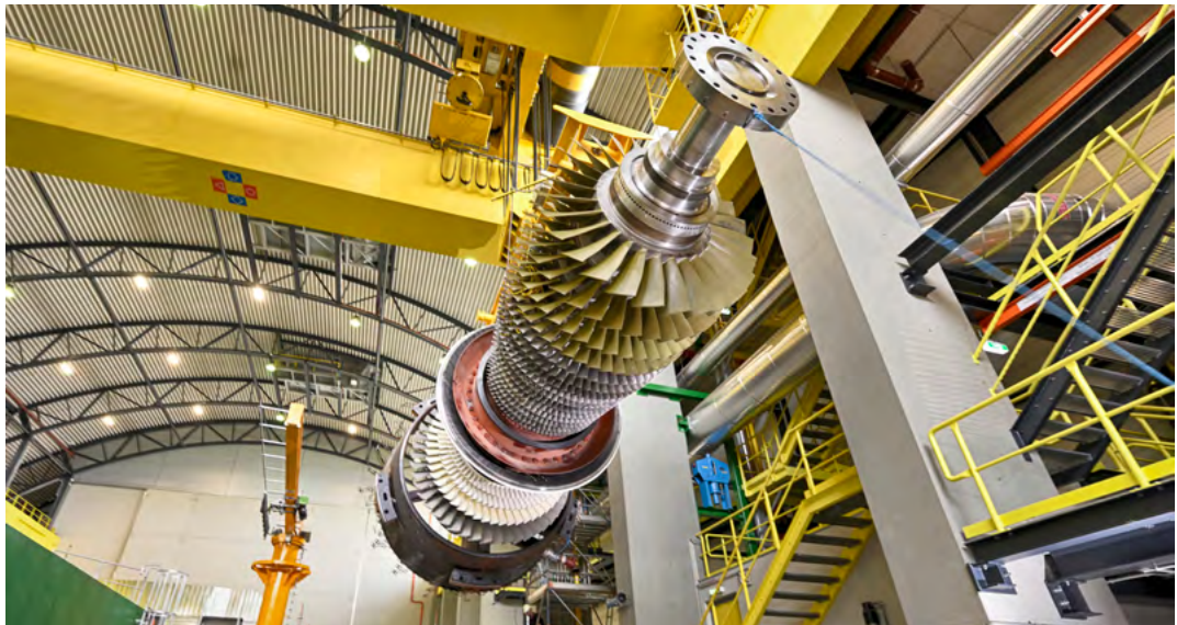
Gas turbine at the Donaustadt power plant site, home to the first-ever trial of cofiring hydrogen for energy generation, Photo: Wien Energie/Johannes Zinner
