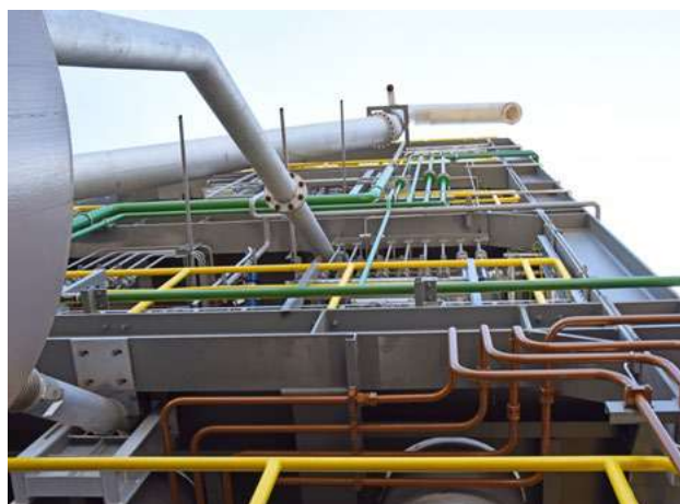
Discharge line to the product cooler, photo: primetals.com
