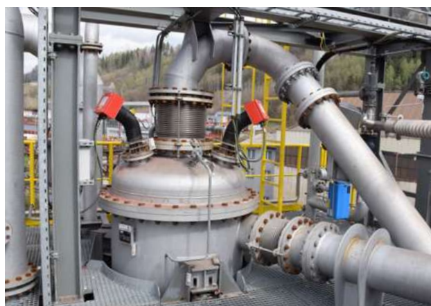
Top ore/DRI bunker, photo: primetals.com
