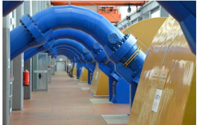
View inside a hydropower plant, photo: TU Wien
