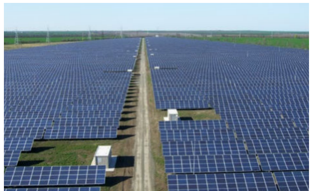
Large-scale PV facility, photo: AIT/T. Krametz
