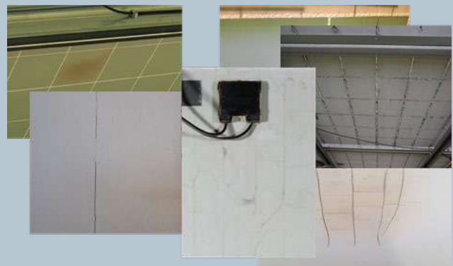
PV modules with defective back skins, photo: OFI
