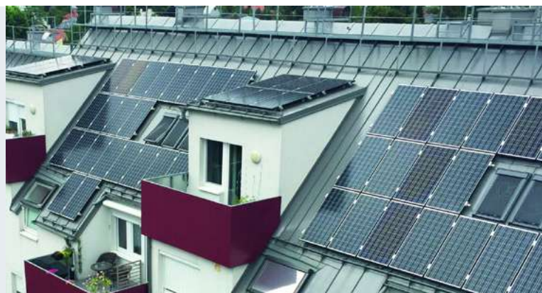
PV facility in Vienna's Stammersdorf district, photo: PV Austria
