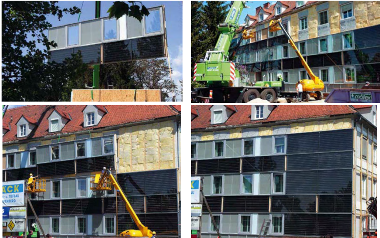
Picture 24: Assembling procedure of the facade modules with integrated collectors. (Source: AEE INTEC)
