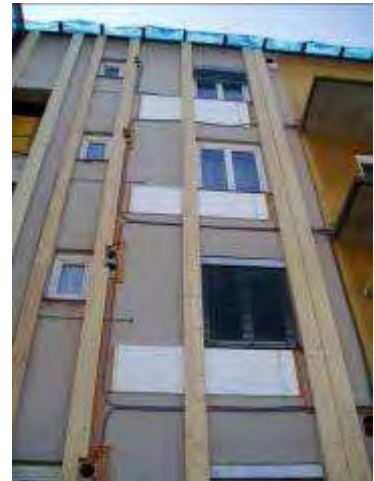
Picture 2: Photo during renovation works on the exterior wall with the levelling laths assembled on and in-between the insulation panels with inserted heating pipes.
