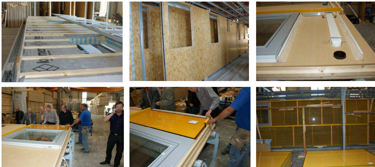
Picture 3: Assembling the prototype in the fabrication of carpentry Kulmer Bau (Source: AEE INTEC)
